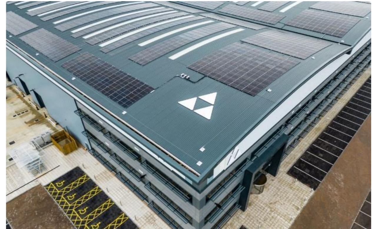
Fig 69. Illustrative example of a PV installation on the roof.
